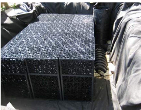
AquaBlox® D-Raintanks® set at foot of self-sustaining waterfall.
