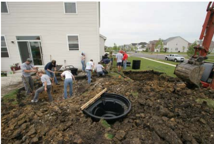
Excavation of site. Rainwater storage basin in background and BioFalls® Filter shown in foreground where waterfall will begin.
