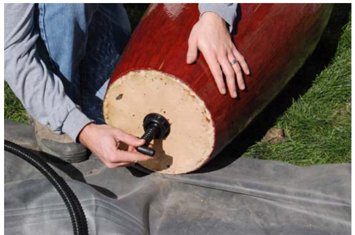
The decorative urn is connected to the plumbing system.
