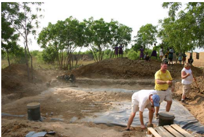
Two feet of soil is mounded over the reservoir to block water born contaminants from entering the basin.
