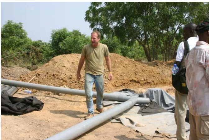
Underground pipe is installed to carry water from the downspout to the rainwater storage basin.
