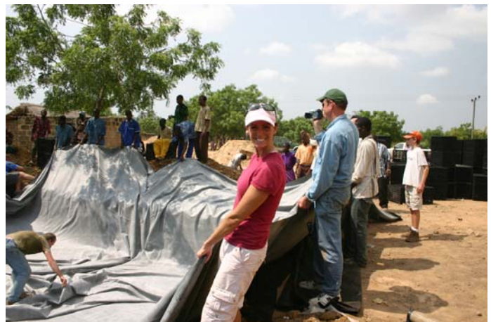
Aquascape Foundation volunteers work with village residents to spread the liner over the basin.
