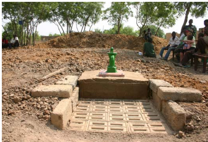
A hand pump is installed where residents will be able to pump clean water from the reservoir.
