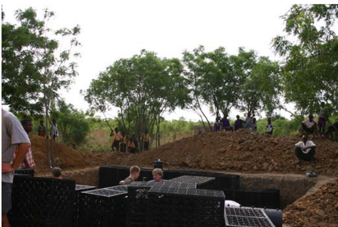
240 AquaBlox® Water Matrix units are set into the basin creating an 8,000 gallon reservoir.
