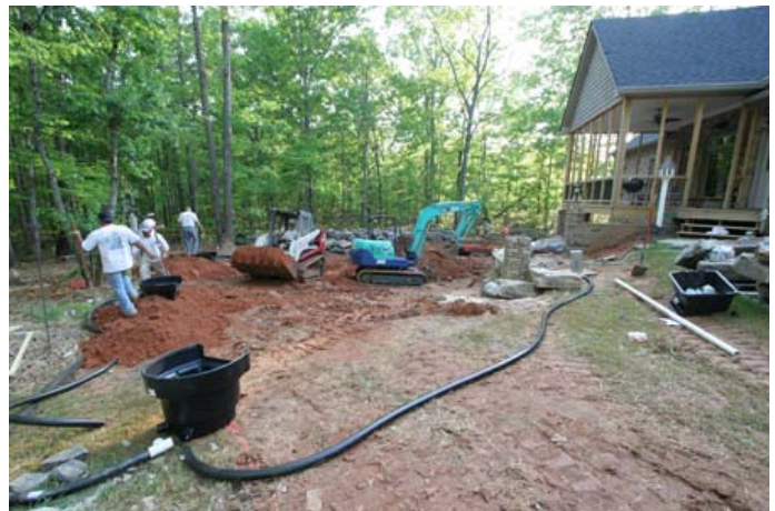
Excavation begins and BioFalls® Filters are placed to mark the start of each of the 3 waterfalls running into the underground basin.
