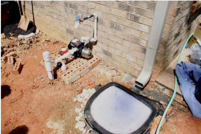
The Downspout Filter is located underneath the gutter and the Booster Pump is ready to hook up to a garden hose for irrigation.
