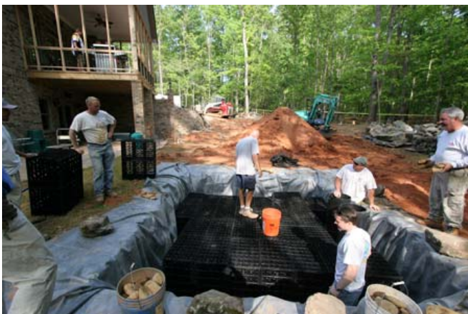
AquaBlox® are set into the storage basin after liner is placed. The 2500 gallon storage area is located at the lower end of the property.
