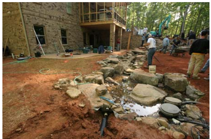
The waterfalls and stream are rocked in and directed toward the underground storage basin, which has also been rocked in.
