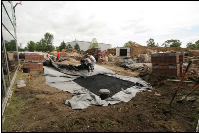
A water permeable woven geotextile fabric covers the top of the AquaBlox® Water Matrix tanks providing a permeable base for the gravel and screening to be spread over the storage system.
